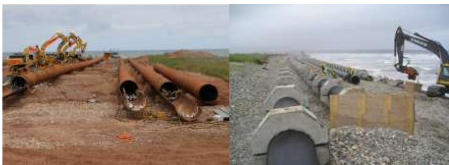
Figure 2.4 Steel (Left) and HDPE (Right) Conduits
